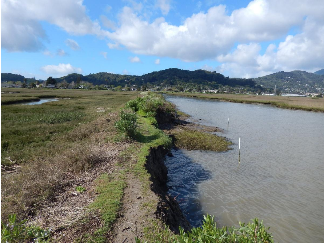
Figure 13.1 Erosion of the levee surrounding Muzzi Marsh, Corte Madera, California. As upstream dams capture sediment and sea level rises, San Francisco Bay's surviving salt marshes are threatened. Photo by Sharon Levy.
